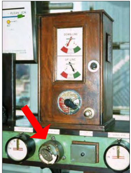
A 'Welwyn' mechanical winder avoids the possibility of a signalman giving a 'Line Clear' in the belief that a train has left the section when it has not, and thus giving a second 'Line Clear' in error.
