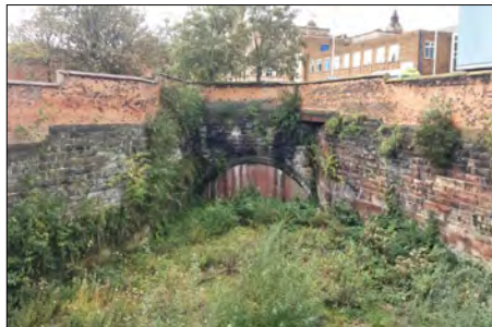
Above : The tunnel portal into Birkenhead Woodside Station viewed from Church Street bridge.
