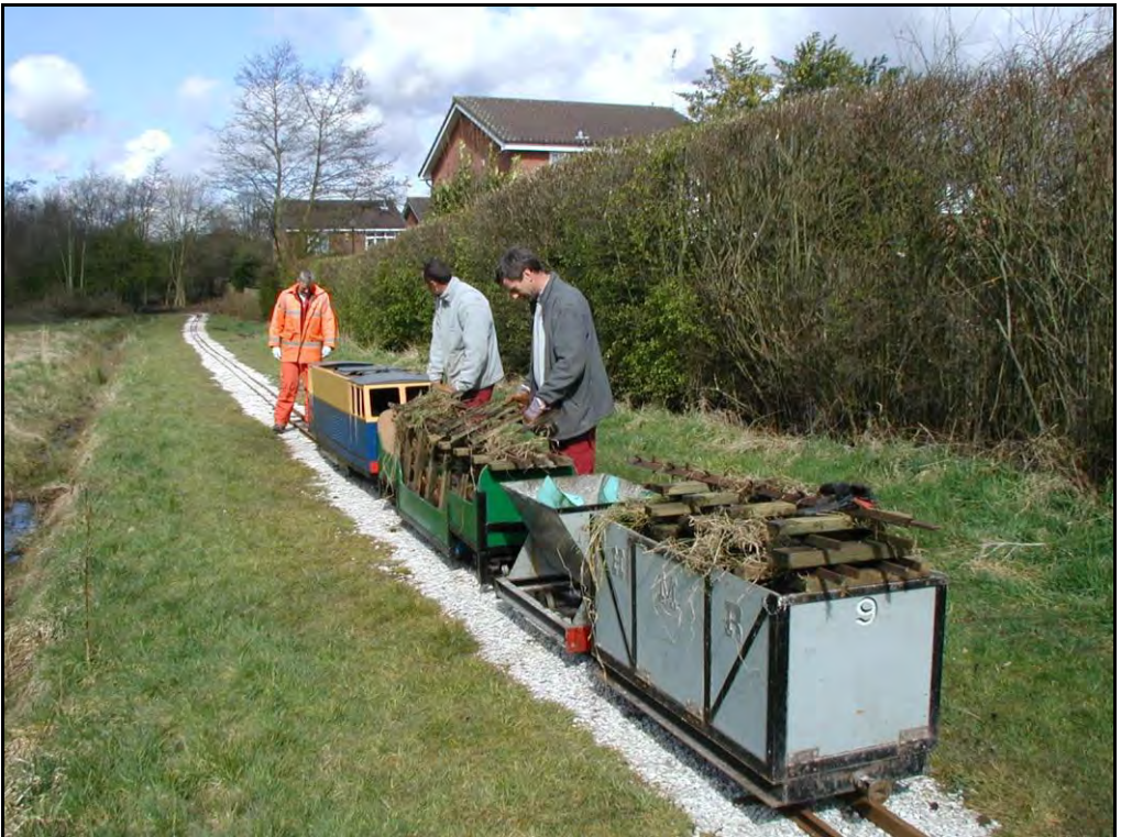
Engineering works on the HMR on 27 March 2008. The section of line at this location was realigned during the winter of 2007/8 and new track was laid. The original track from the early 1980s was being removed from site by a works train. Photo by Paul Wright
