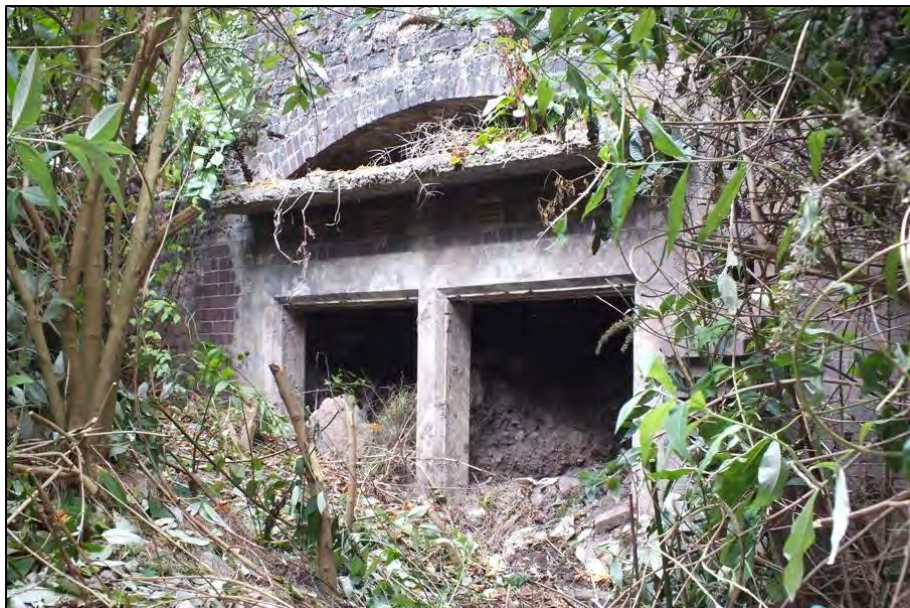
The remains of Park Lane signal box seen during the 8D visit to the Wapping tunnel on 17 th October 2015. Photo by Tony Foster
