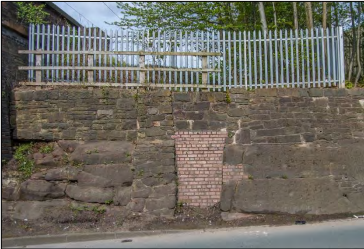
Looking across Helena Road at the bricked up aperture which formed the station entrance. A welcome addition for the weary miner travelling home from work. Photo by Terry Callaghan
