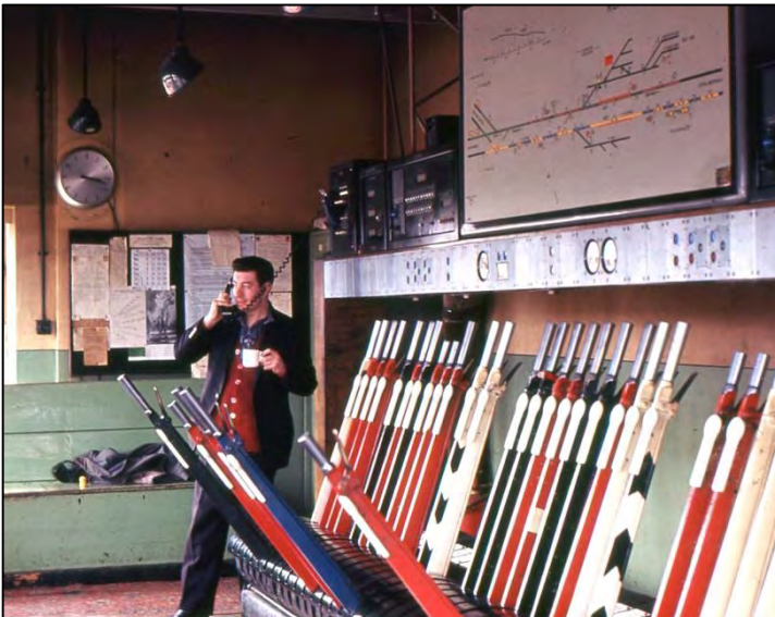
A view from inside Runcorn signal box taken in the early 1960s. The box controlled the junction between the main line and the Folly Lane branch. The track layout as it would have been at the time of the 1965 crash is seen above the levers.
