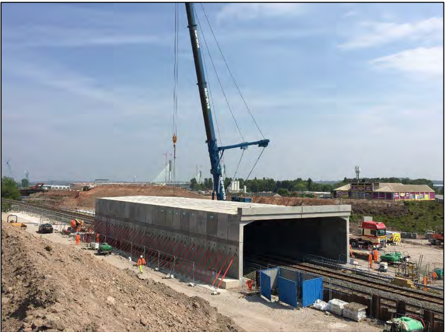
The new bridge over the Widnes deviation line was taking shape when this view was taken on 12 th May 2017. The bridge is part of the Mersey Gateway scheme and it is the only overbridge on the deviation line (the bridges that form part of the Silver Jubilee Bridge route being located at a point that was part of the original 1852 Warrington & Garston line). Photo courtesy of Merseylink
