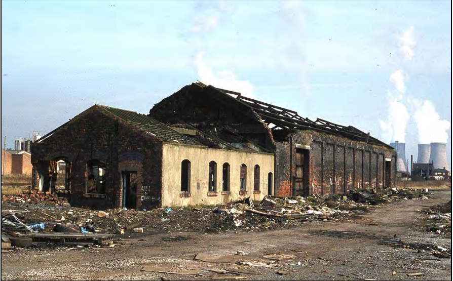
The derelict goods shed at Tanhouse Lane seen on Monday 3 March 1980. The shed had last been used in the early 1970s by British Road Services. They had started an operation from Tanhouse Lane after it had closed to public goods by rail. Less than two years after this photo was taken rails were laid on the site of the goods shed as part of a new connection that was put in to the Widnes deviation line. That connection allowed the 1961 chord connection to the St Helens line to close. Photo by Brian Roberts
