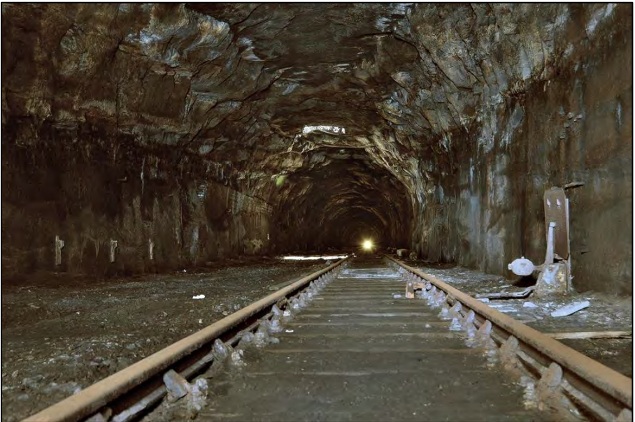
The long shunting neck inside the Victoria tunnel looking west on 15 June 2015. The light in the distance is from the Byrom Street cutting which is where the western portal of the Victoria Tunnel is located. To the right of the photo a tunnel gong can be seen. Photo by Terry Callaghan
