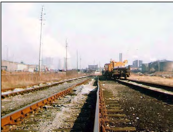
Left: Tanhouse Lane yard was in poor condition when this view was taken in February 1982. The view is looking east from the western end of the yard. The main line had been to the right of the sidings. Photo by Paul Wright
