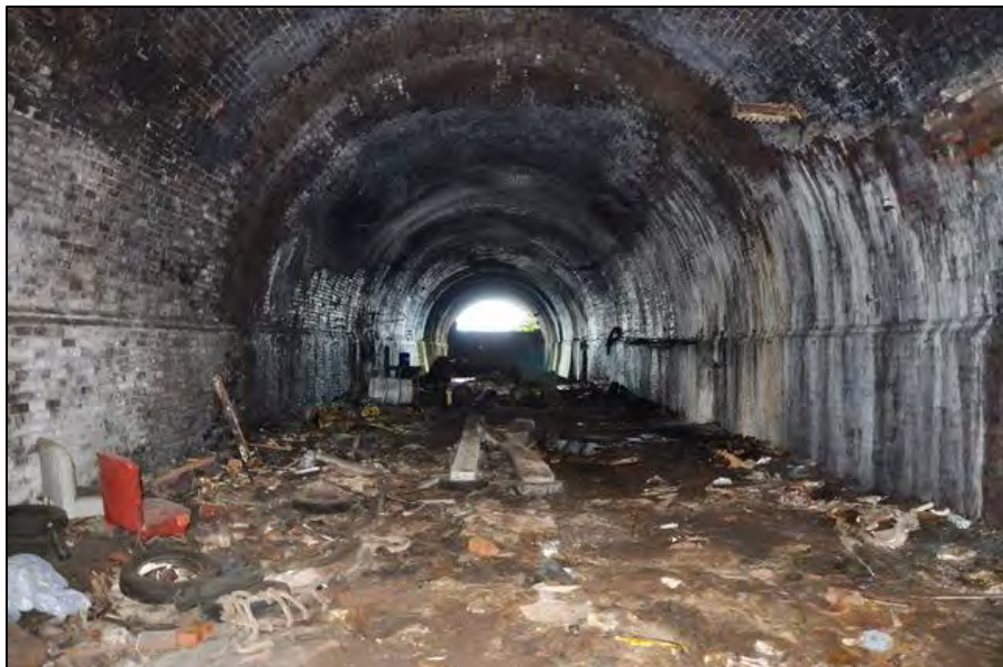
Looking north-west along the Dingle LOR tunnel on 10 July 2018. The western portal of the tunnel can be seen in the distance. Photo by Doug Birmingham
