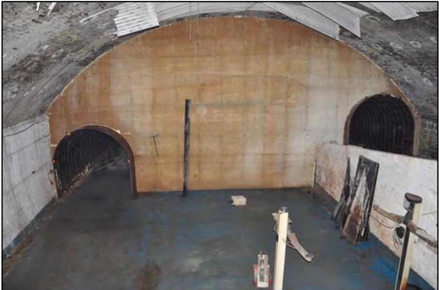
The concrete support that was built to secure the tunnel roof seen on 10 July 2018. Photo by Doug Birmingham
