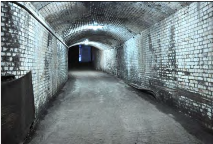
Left: Looking towards street level along the pedestrian access subway of Dingle (Liverpool Overhead Railway) station on 10 July 2018. Photo by Doug Birmingham
