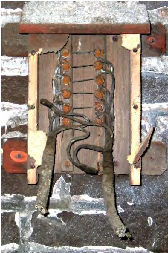
Left: Electrical Signalling equipment from the Liverpool Overhead Railway can still be seen inside the Dingle Tunnel. This view was taken during the 8D Association visit of 10 th July 2018. Photo by Tony Foster
