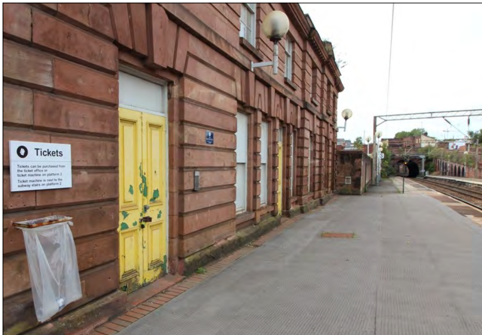
The poorly maintained doors (note the two-toned paintwork) at the left of the photograph mark the position of the Edge Hill station foreman's office in the 1960s. Used by foremen Bill Harrison and Sid Wightwick, the office also contained a train describer. Photograph by Dennis Flood
